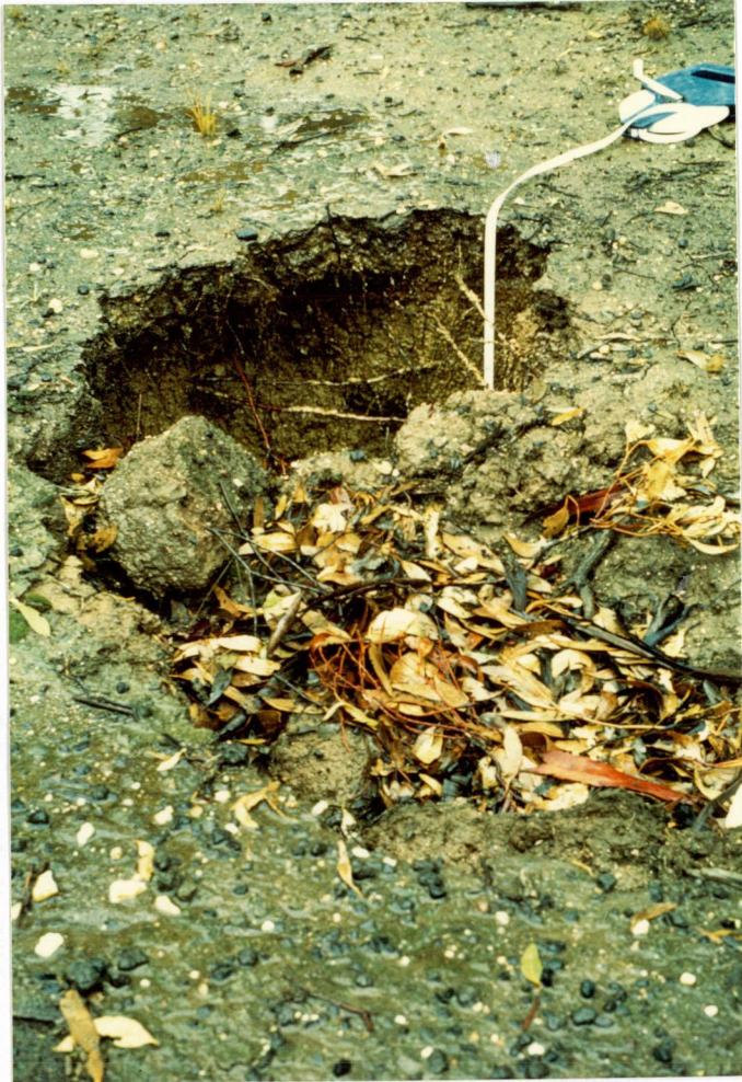
Plate 7 'Sinkhole' (photographed in road reserve, Spring 1983)
